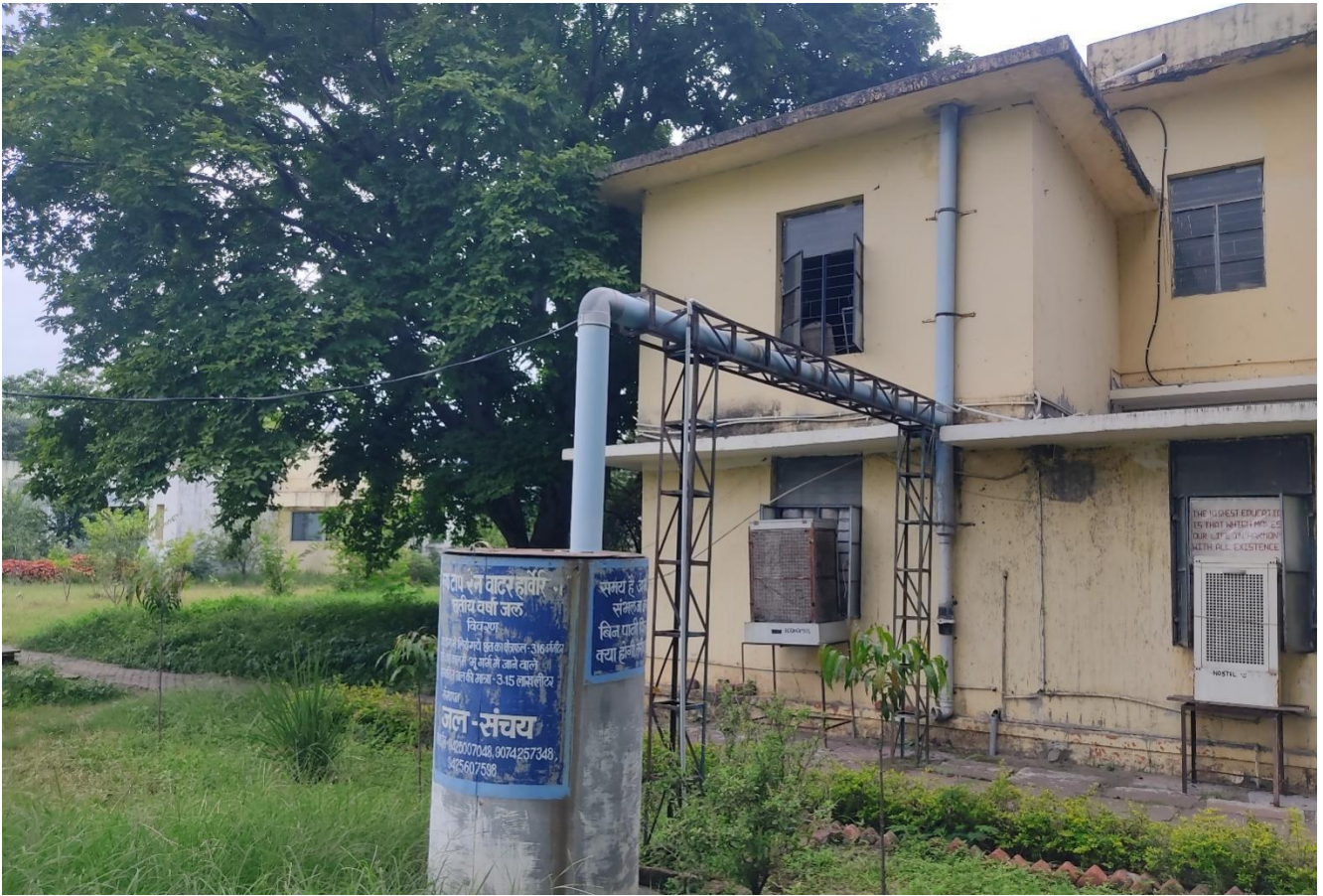
Figure 14 Rain water harvesting system
