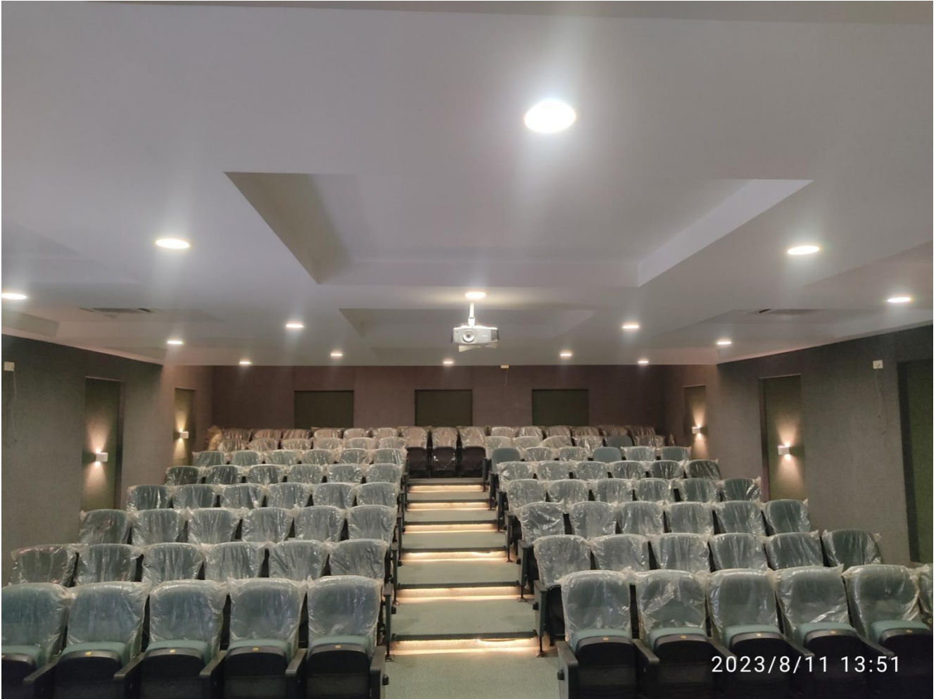
Figure 8 LED Lighting fixtures
