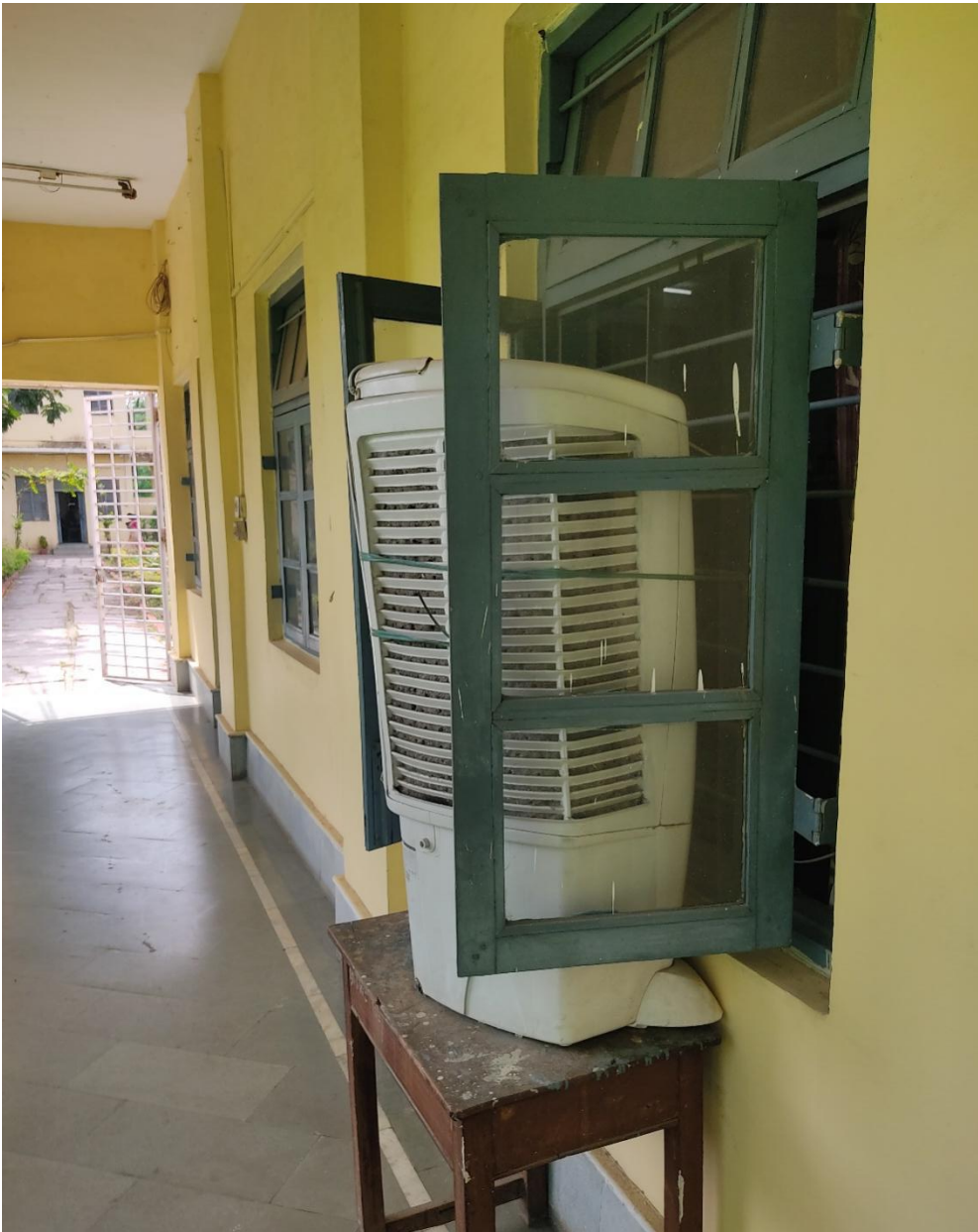
Figure 10 Air Cooler installed in the premises
