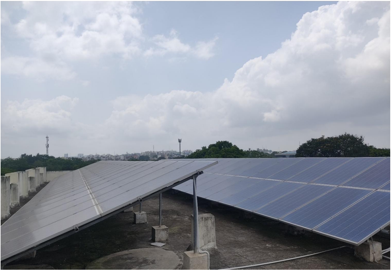
Figure 5 Solar Panel installed at the premises
