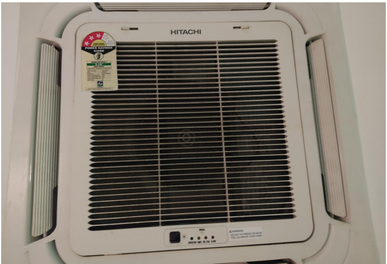
Figure 11 - Star rated Air conditions installed
